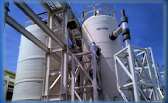
Fluidized Bed Bioreactor at PNNL's 200-W P&T Facility (right)
